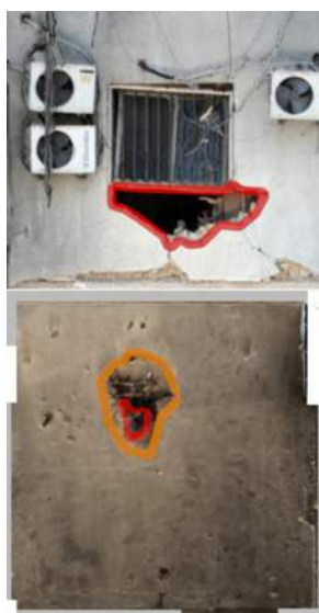
Figure 22: Alignment between perforations (red) to the façade of floor ten, and the ceiling of Bedroom 3 on floor nine.
