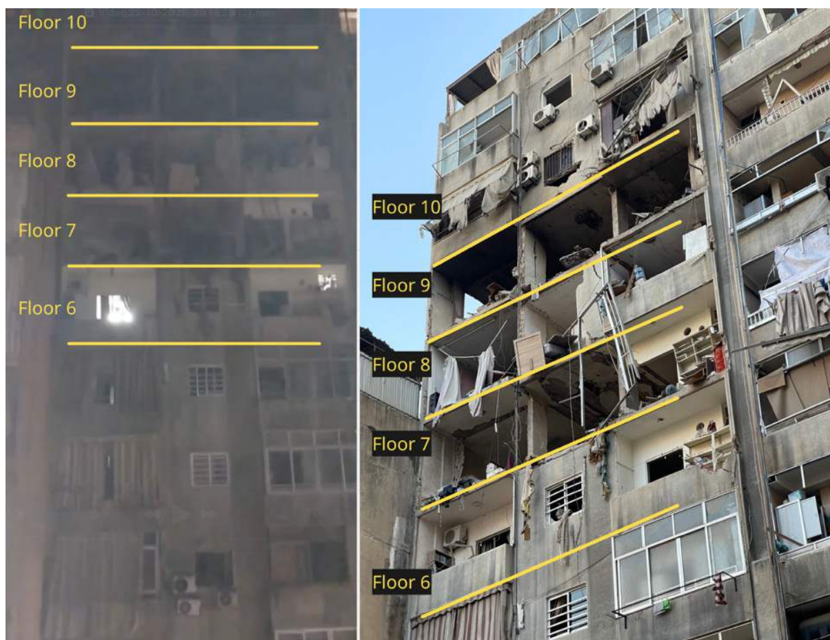
Figure 12: Photographs from 26 November (left) and 5 December (right) show damage sustained to the north façade of the Cherri building.
