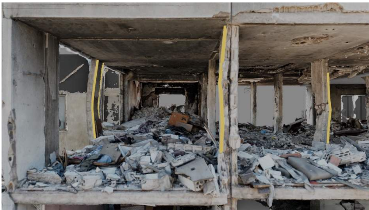
Figure 15: View into Bedroom 2 of the Cherri flat from the north, with deformation marked.
