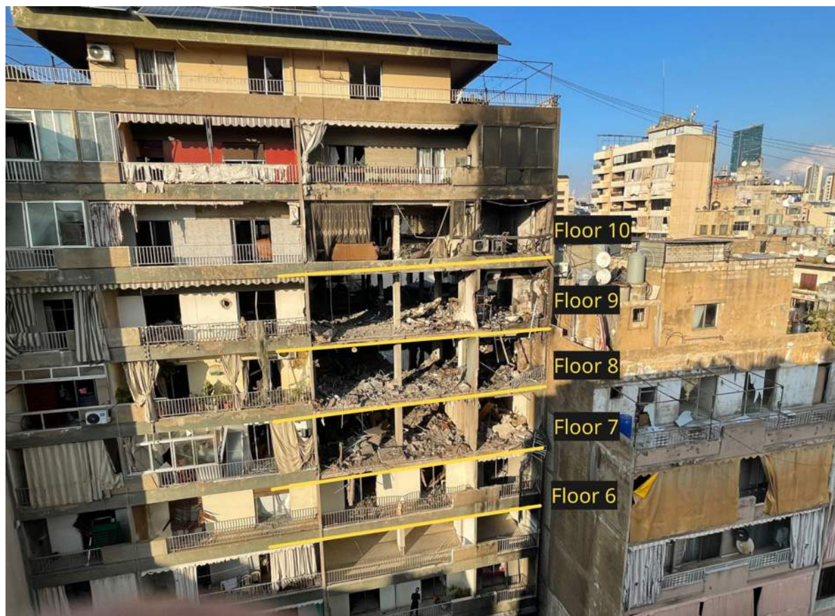
Figure 11: Photograph from 5 December 2024 showing damage to the south façade of the Cherri building.
