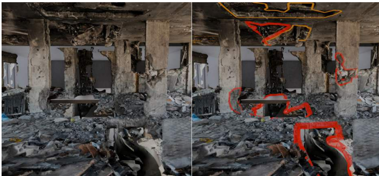
Figure 4: Before (left) and after (right) annotation of perforations (red), and surface damage (orange).
