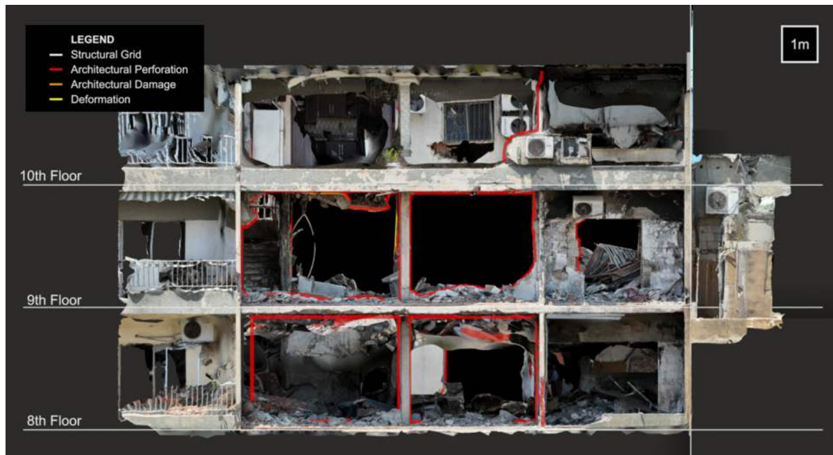
Figure 10: Photogrammetry model showing damage sustained to the south façade of the Cherri building.
