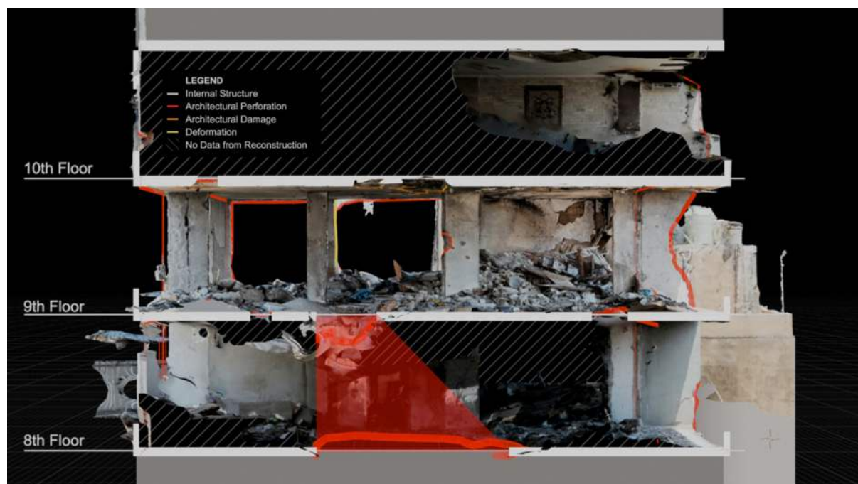
Figure 25: Alignment between perforations in the TV room on floor eight and nine.
