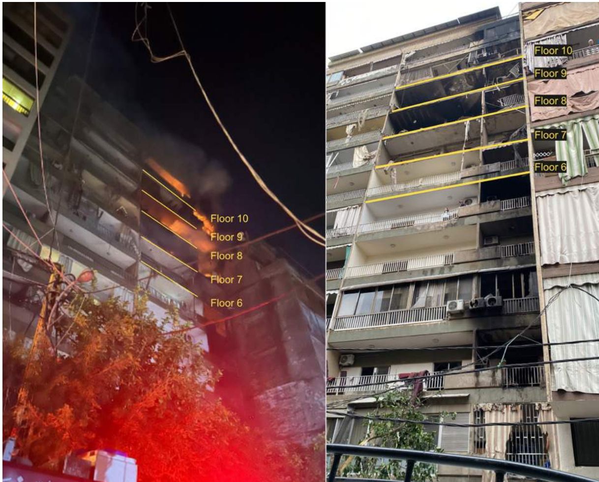
Figure 9: Documentation from 26 November 2024 (left) and 27 November 2024 (right) showing fire and burn marks on the south side of the Cherri building.
