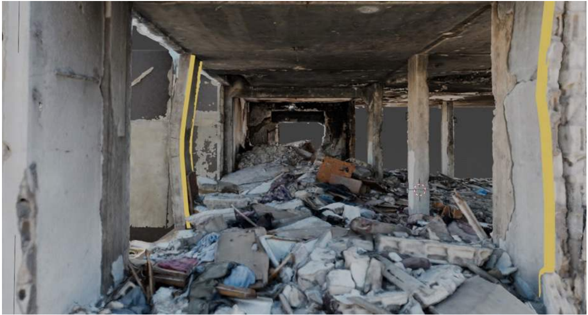
Figure 27: Close up of Bedroom 3 in the northeastern corner of the Cherri flat, with deformations to structural columns marked in yellow.
