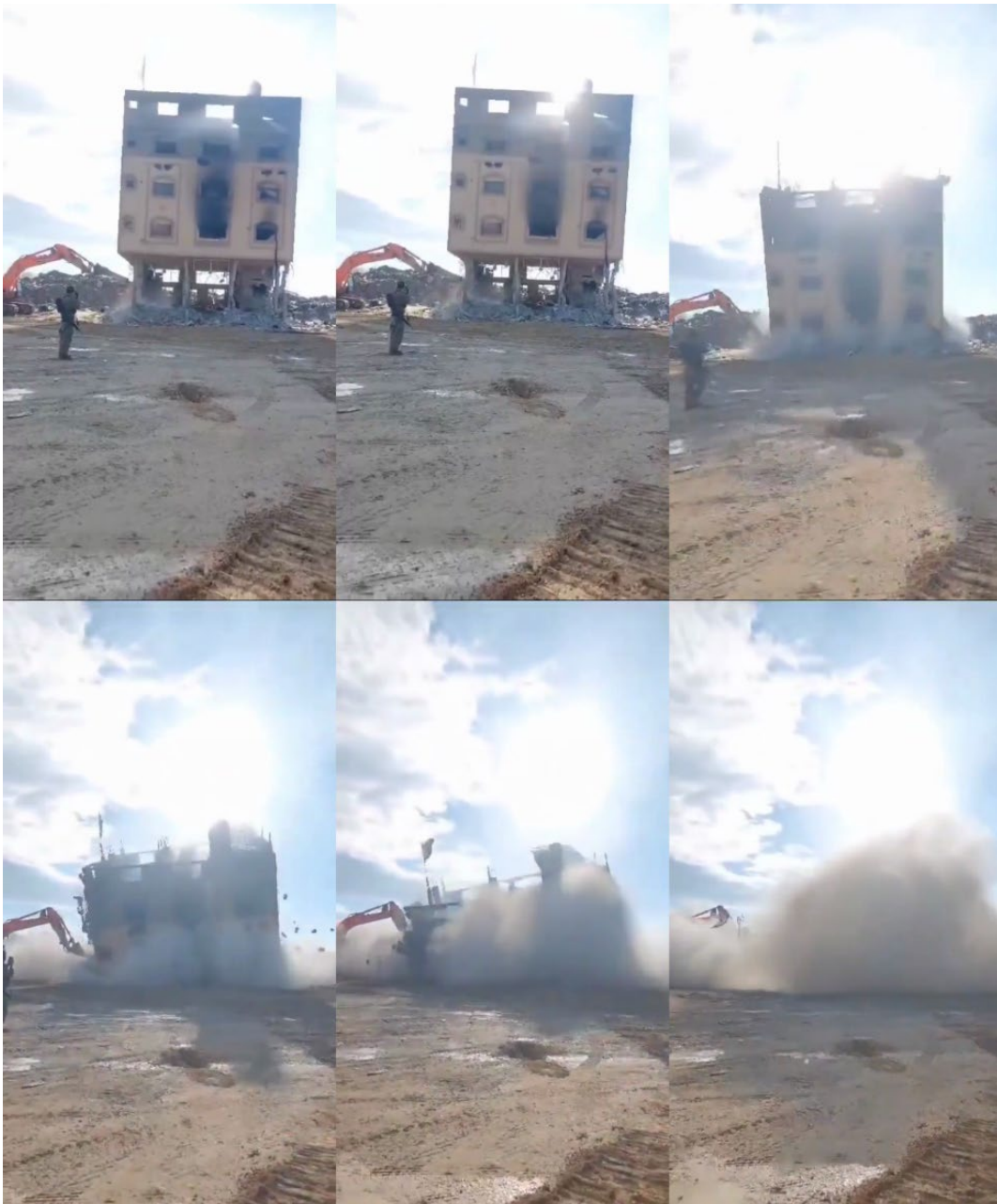
Figure 9 : Frames of video of the demolishing of building in Netzarim Corridor on 24 January. [ID: 50124-53431]
