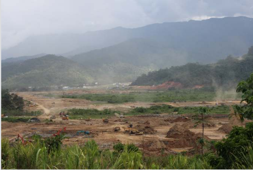
Img: Construction of the tailing dams in the former site of the San Marcos village, January 2016
